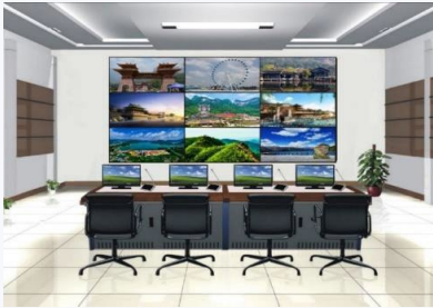
Video Intercom Management Controller Duty room, emergency command center
