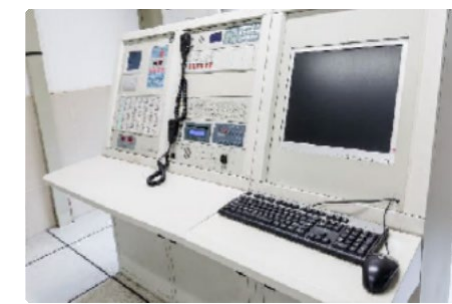
Third-party docking (fire fighting/CCTV)
